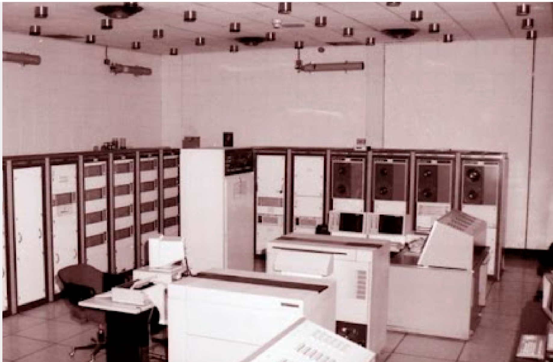
Computers Room COC/SOC Torrejón (1976)
